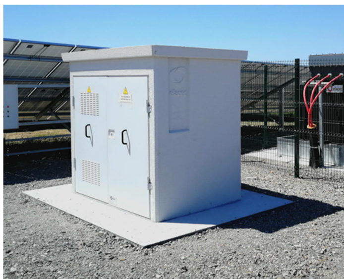
Photo 2-12: Typical cabin indoor switchgear used in the ‘outdoor solar station solution’ (as per Solar Station Option A)
