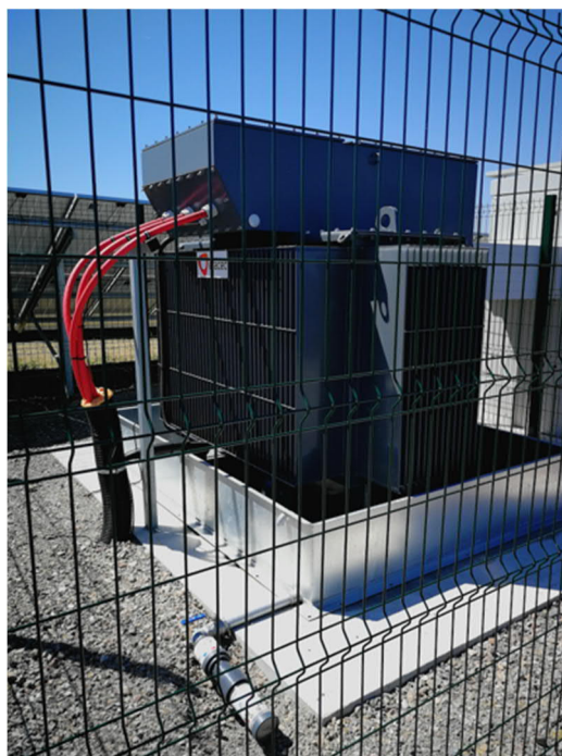
Photo 2-10: Typical outdoor transformer (as per Solar Station Option A)
