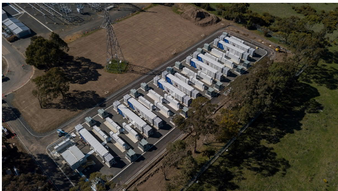
Photo 2-13: Typical battery storage compound configuration ( image reproduced courtesy of Fluence Energy )
