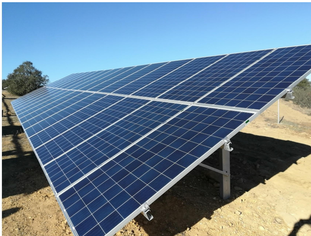
Photo 2-3: Solar panels with south facing configuration
