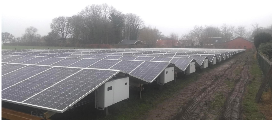
Photo 2-4: Solar panels with east-west facing configuration ( image reproduced courtesy of Huawei )
