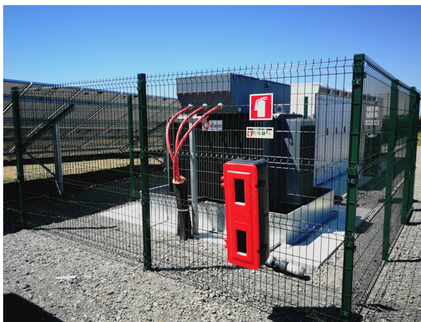
Photo 2-15: Typical transformer compound fencing
