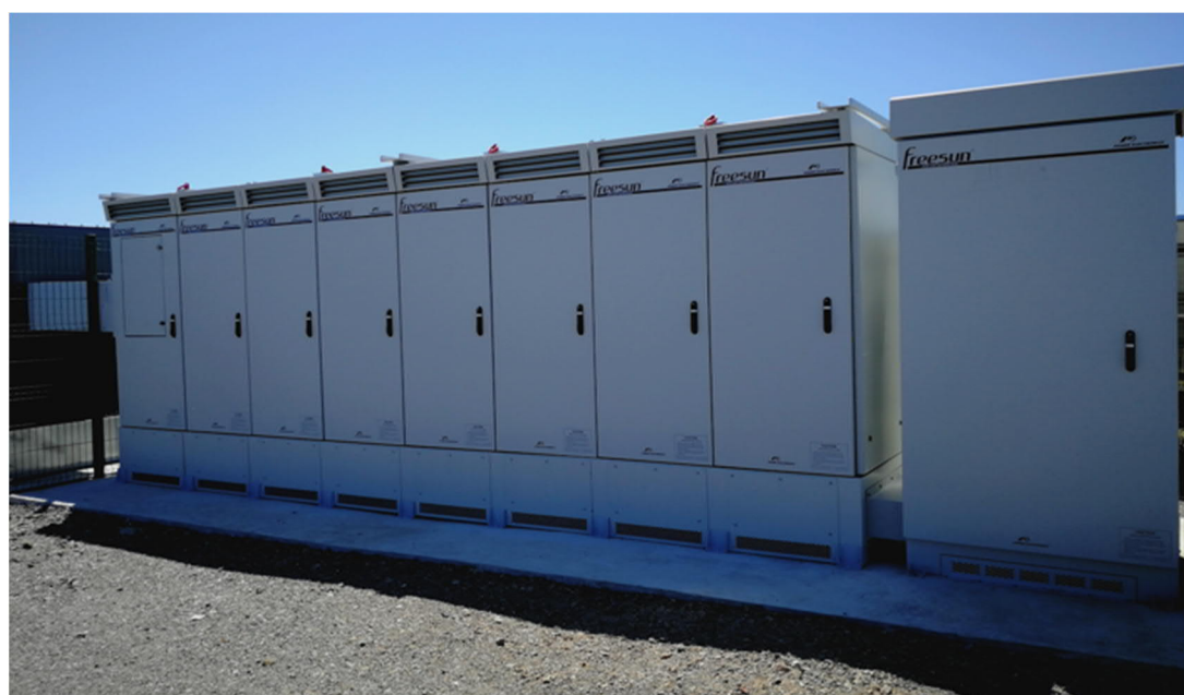
Photo 2-8: Typical outdoor centralised inverter (as per Solar Station Option A)
